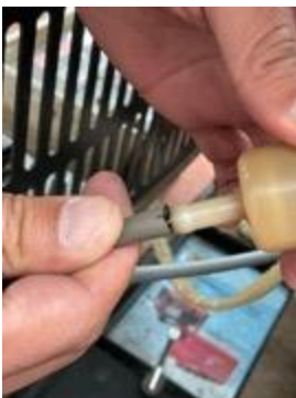
The generator has a small rubber tube for gasoline and it has broken. This is due to dryness and years of use. We'll buy it in town.
